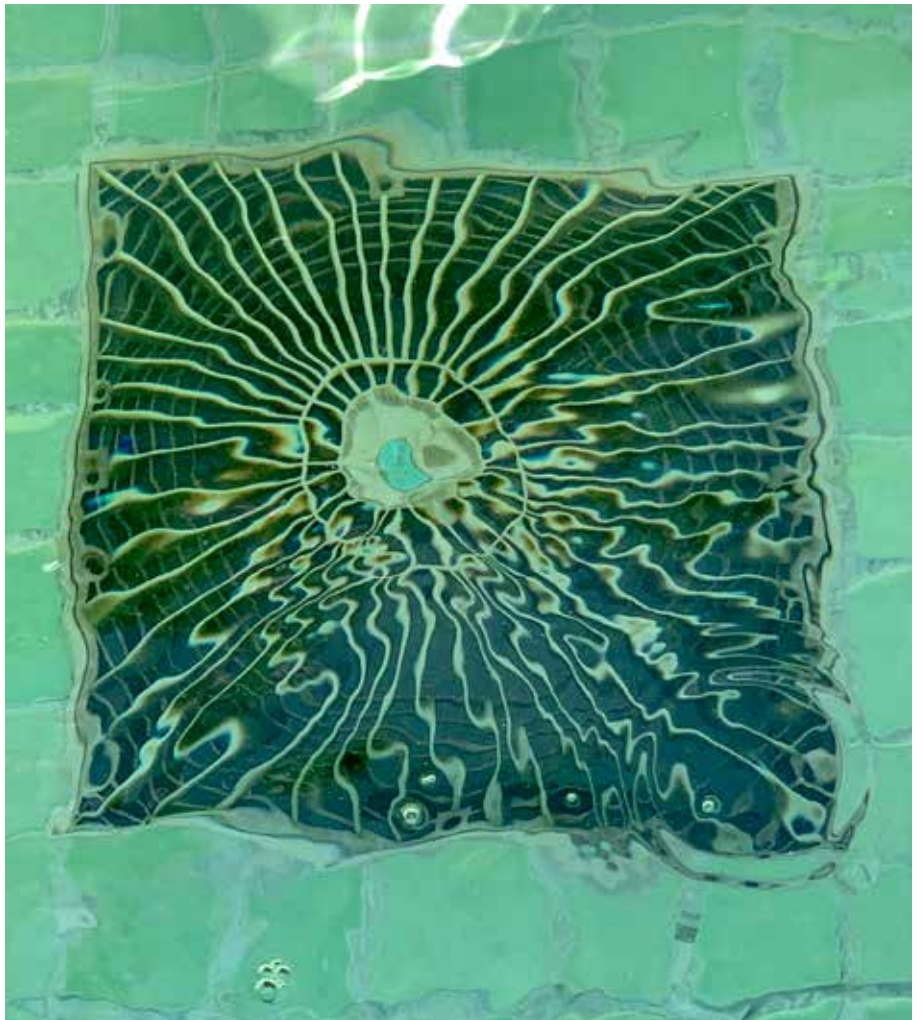
Hot Tub Drain San Ysidro Ranch, Montecito Lawrence Bridges
